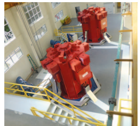
▼ Unit hall at HPP Sabangan
