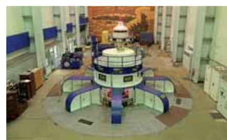
▲ Unit 1 and 2 at Iovskaya hydropower plant
